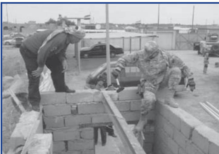
Sgt. Ernest Spycher of Reston, a soldier of the 266th MP Co. assists one of the Al Hartha Iraqi police with construction of a rooftop. (Courtesy of 266th Military Police Company).
